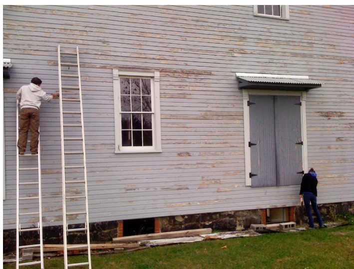
The west side of the Darden Mill (facing the train tracks) in Elkins is getting a paint job. Here Hands-On Team Members Blake Crow and Katie Booth are scraping as they prepare to paint. Photo: Scott Prouty
