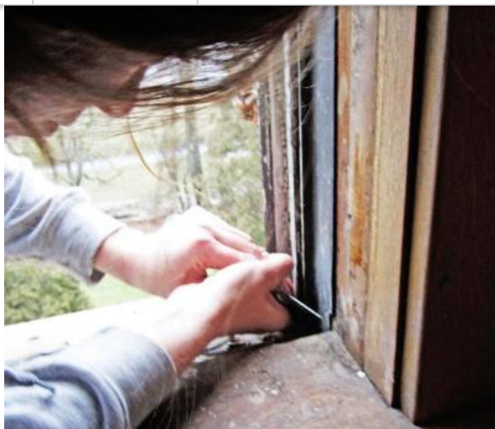
Beckerle assists with removing a historic window sash from the Kump Education Center for re-glazing and repair.
