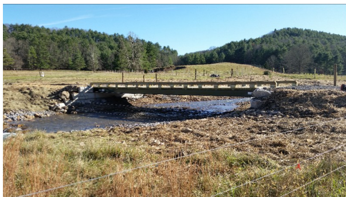
After shot of low water bridge replacement. Photo by AFHA AmeriCorps member Travis Ferry
