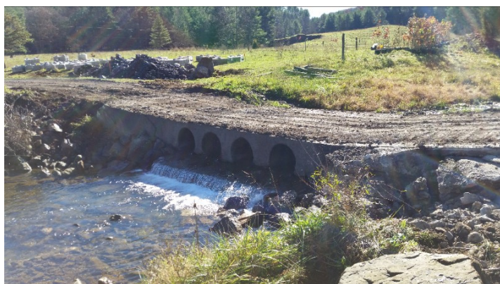
Before shot of low water bridge replacement. Photo by AFHA AmeriCorps member Travis Ferry
